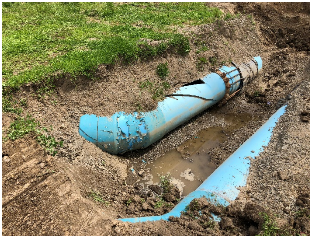
Photo #3 CT Chamber Rupture Starting @ Joint Restraint
