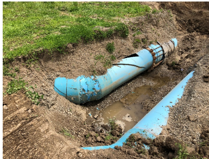
Figure 3: Discolored and Blistering Pipe
