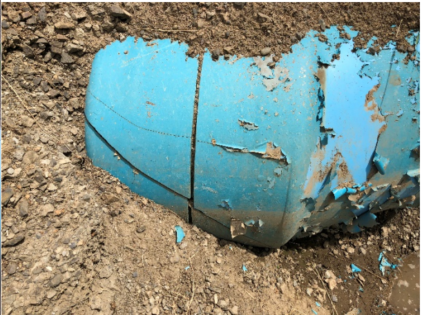
Photo #6 Peeling of Sun Bleached Pipe @ Bend Exhibiting Failure
