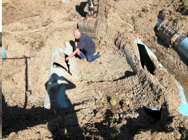
Photo #2 Excavated CT Chamber after Rupture
