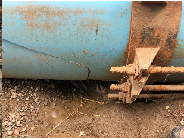
Photo #4 Close up of Rupture Starting @ Joint restraint
