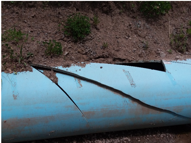
Photo #5 Typical Pattern of Hoop Stress Fracture
