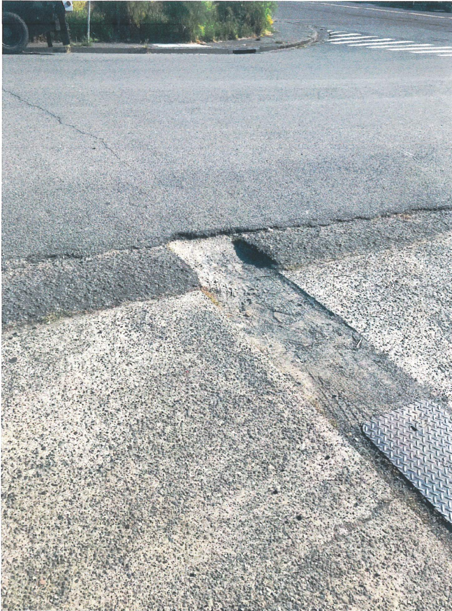
PHOTO OF THE DANGEROUS CONDITION
