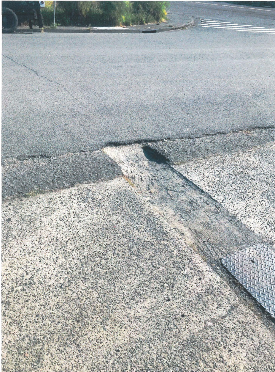
PHOTO OF THE DANGEROUS CONDITION
