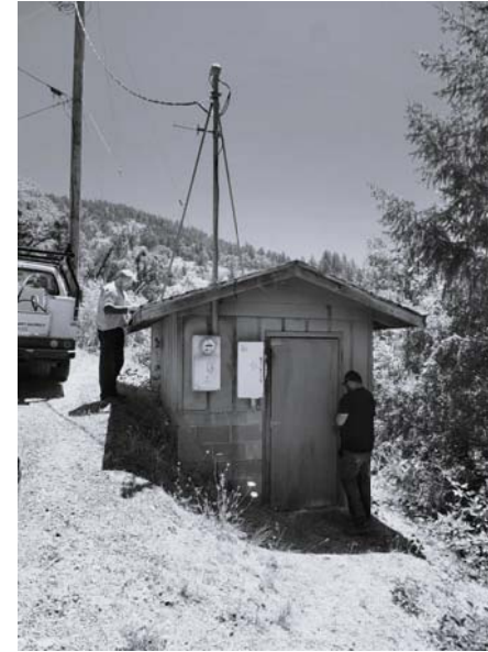
(E) METER/MAIN PANEL & MTS A PHOTO
